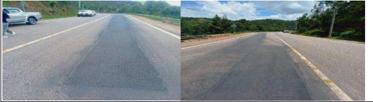
Photo showing repaired patches along the road section at PK 0+000-50+350 as example . Photo taken by OAG on 15/11/2023
