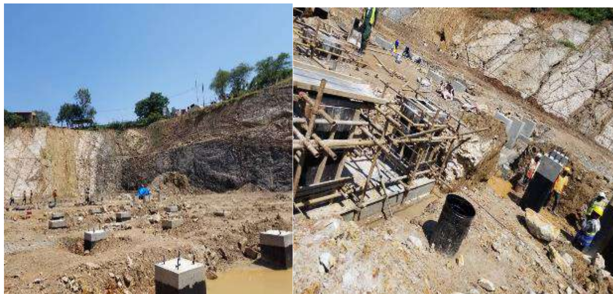
Photos taken by OAG on 29 September 2023 showing works in progress for the construction of Bwishyura substation in Karongi District.
