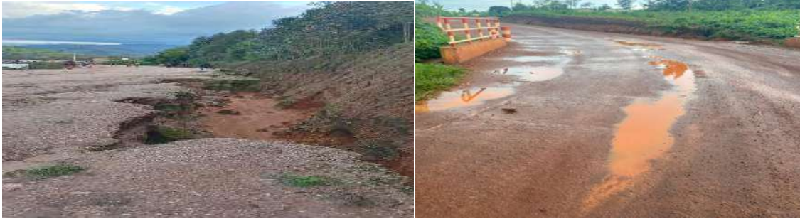
Road pavement deteriorated due to water run-off at PK 18+240: Photo taken by OAG on 17th November 2023 on Nyaruguru feeder road Deflection developed on road surface at PK 0+300. Photo taken by OAG on 17/11/2023 on Gatsibo feeder road
