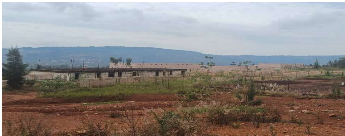
Stalled works of development affordable houses and not being used for the intended purpose: Photo taken by OAG on 23 March 2024.
