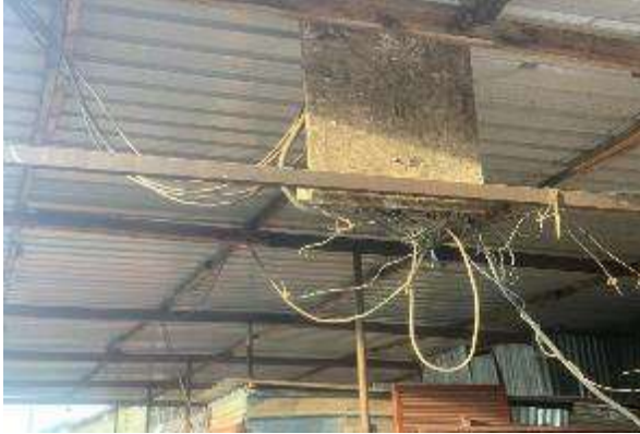
Photo taken by OAG on 11 October 2023, showing the inappropriate electrical installation in Kimironko ICPC
